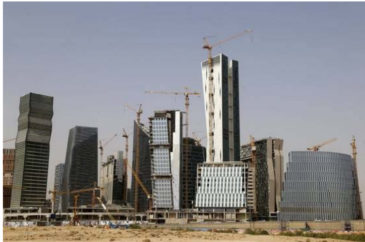
Construction of the King Abdullah Financial District in Riyadh, the Saudi capital. A Saudi family is suing J.P. Morgan over a soured business relationship. FAISAL NASSER/REUTERS
